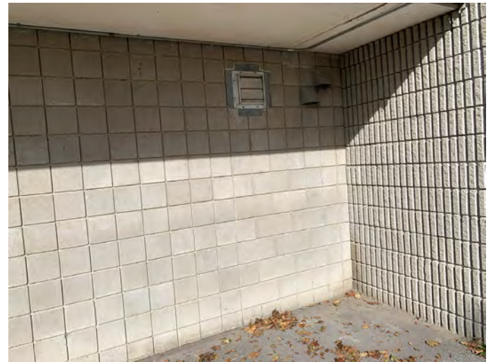
Photo 56 - West Elevation Block Wall Efflorescence
