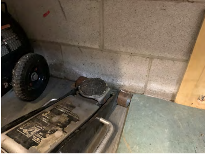
Photo 21 - Masonry Block Wall Efflorescence
