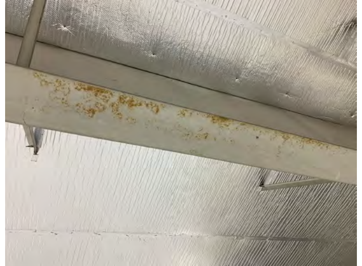
Photo 02 - Pre Engineered Frame Bottom Flange Corrosion
