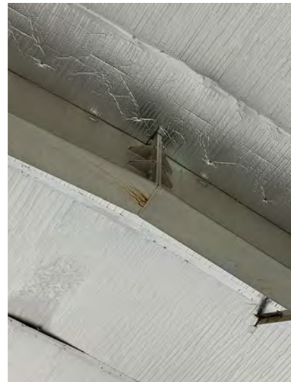
Photo 08 - Pre Engineered Frame Moisture Staining
