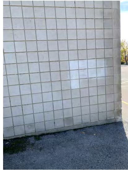
Photo 44 - East Elevation Block Wall Efflorescence
