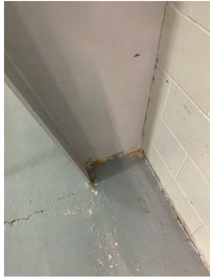
Photo 10 - Pre Engineered Frame Base Corrosion
