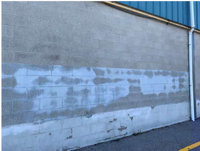
Photo 39 - South Elevation Block Wall Efflorescence
