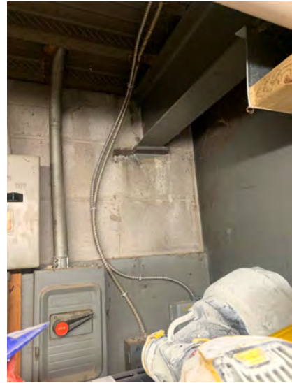
Photo 24 - Masonry Block Wall Efflorescence
