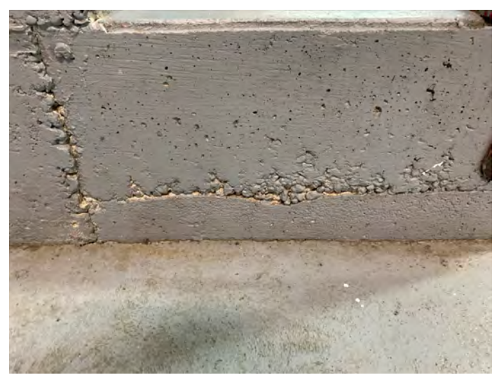
Photo 16 - Bleacher Seating Honeycombing
