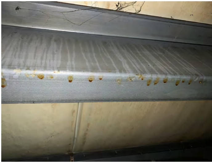
Photo 35 - Partial Second Floor Z Girt Water Staining
