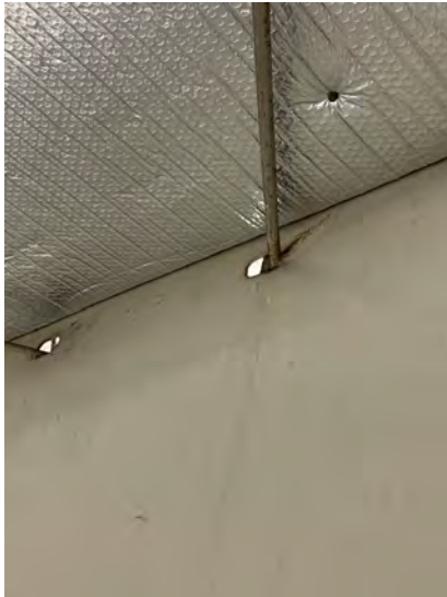
Photo 15 - Pre Engineered Frame Bracing Corrosion
