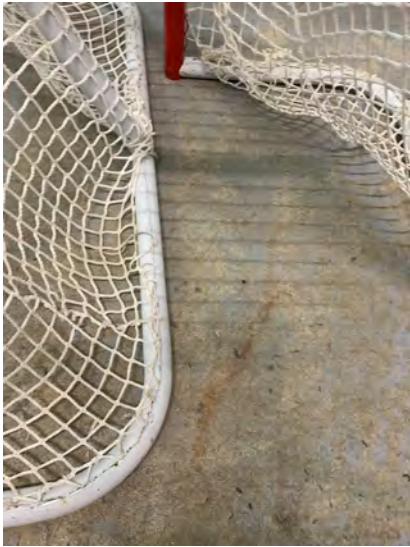
Photo 33 - Concrete Apron Slab Deterioration
