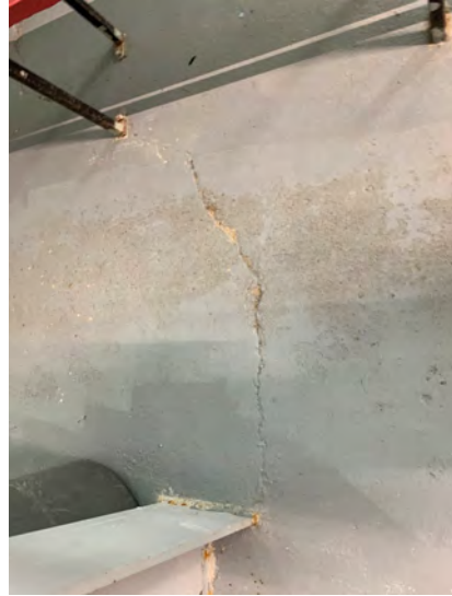
Photo 18 - Bleacher Seating Cracking
