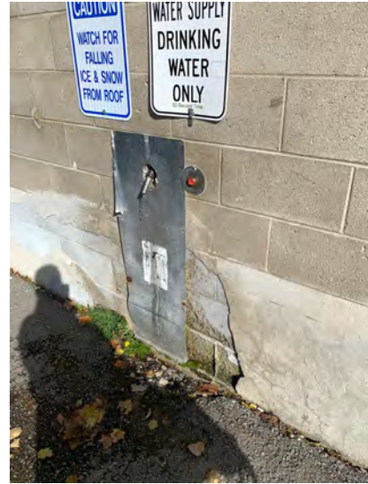
Photo 50 - North Elevation Vegetation and Deteriorated Parging
