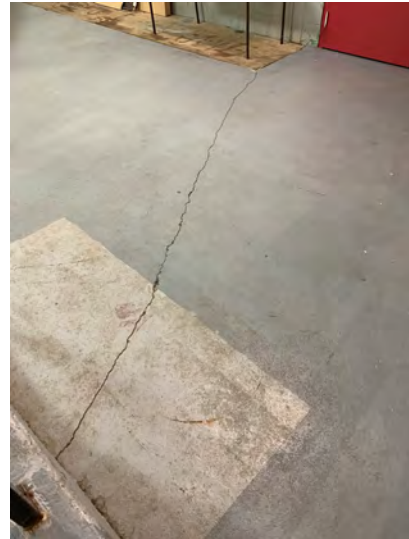
Photo 28 - Concrete Apron Slab Cracking
