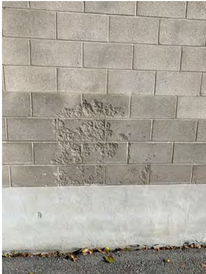
Photo 51 - North Elevation Deterioration
