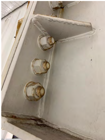
Photo 07 - Pre Engineered Frame Bolted Connection Corrosion
