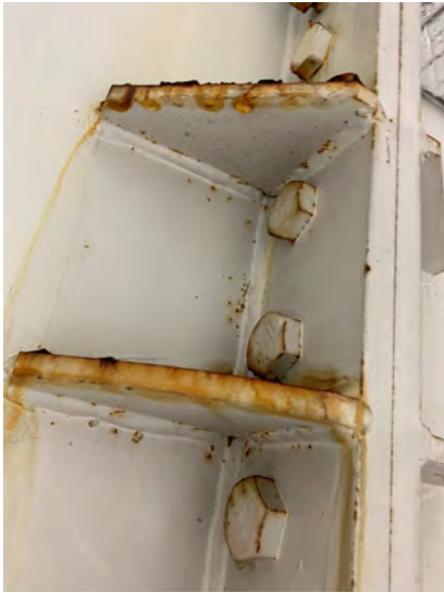
Photo 05 - Pre Engineered Frame Bolted Connection Corrosion
