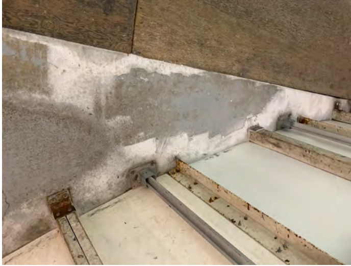
Photo 29 - Concrete Apron Slab Efflorescence
