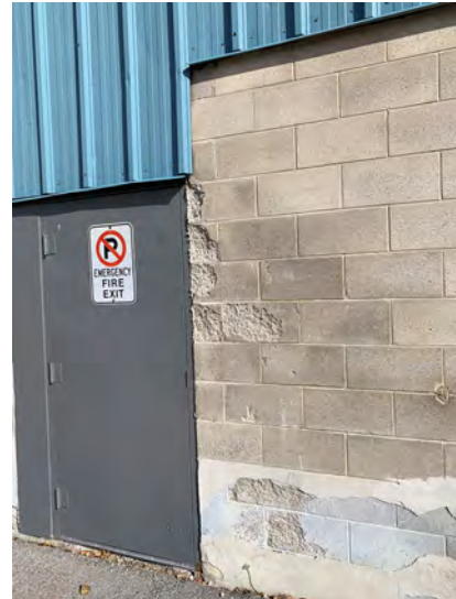
Photo 52 - North Elevation Deterioration 2
