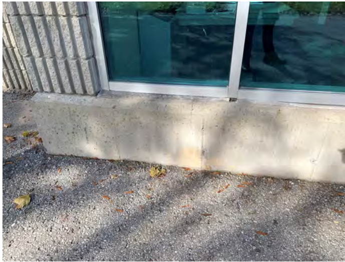
Photo 55 - West Elevation Foundation Wall Vegetation and Efflorescence
