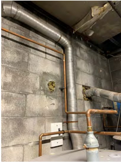
Photo 23 - Masonry Block Wall Efflorescence
