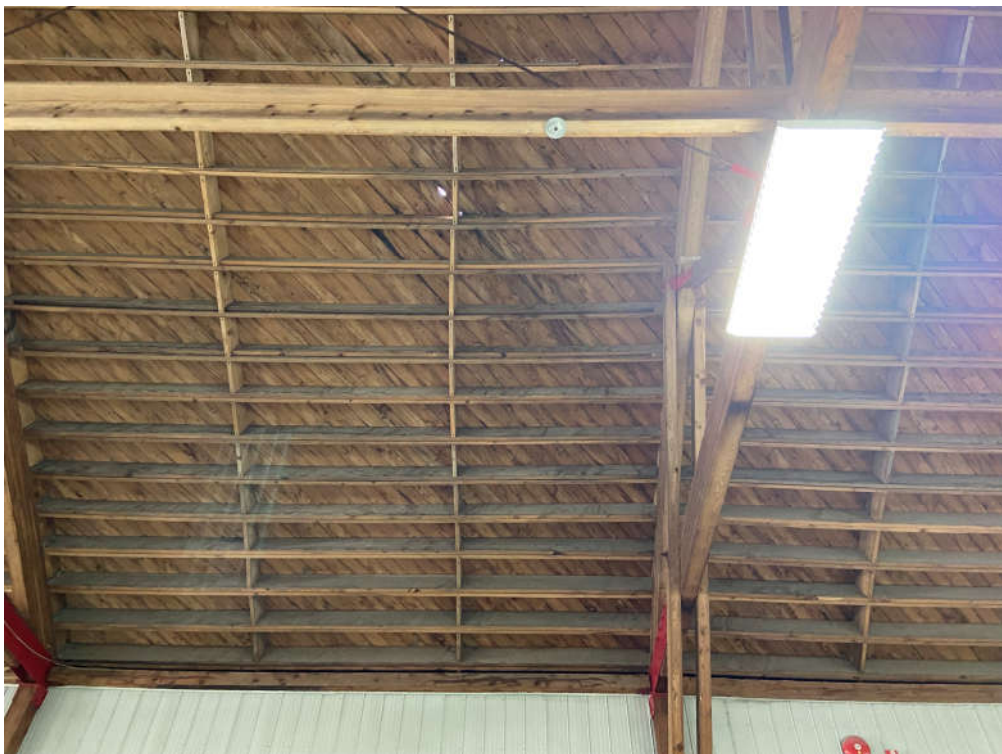
Photograph 4: General area of ant damage seen from below
