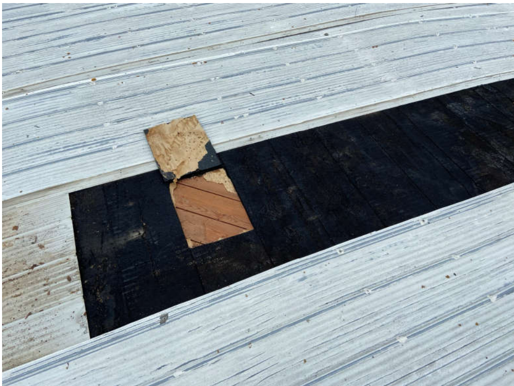
Photograph 12: Close-up of exposed roof deck at north end of building
