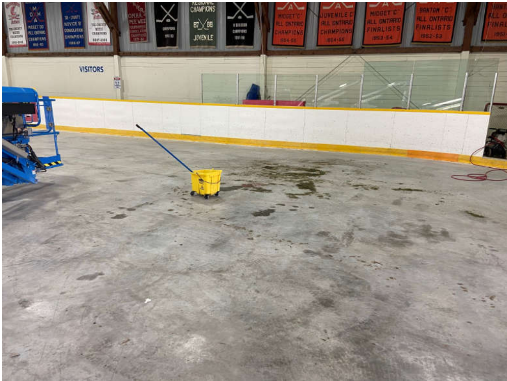
Photograph 2: Reported roof leak at south-east corner of the building
