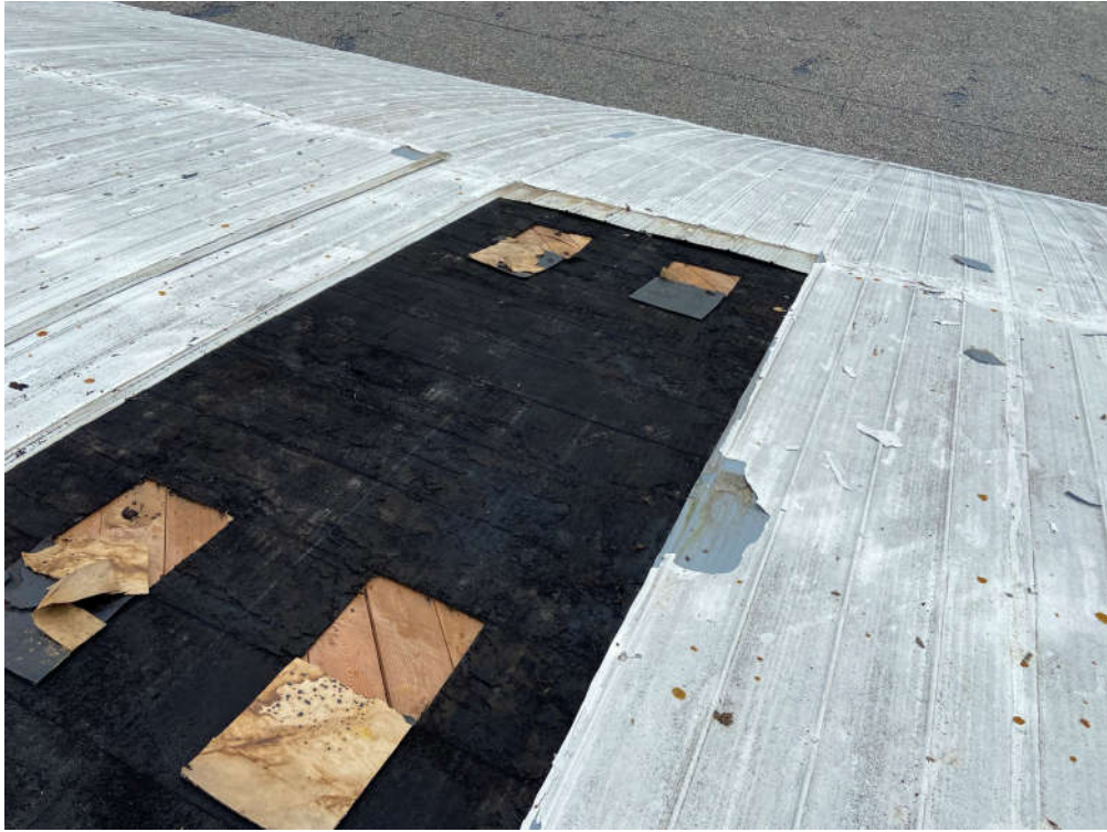
Photograph 9: Roof deck exposed at reported roof leak at south-east corner of building
