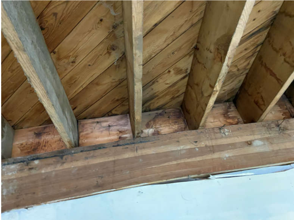
Photograph 3: Area of water staining at north end of arena
