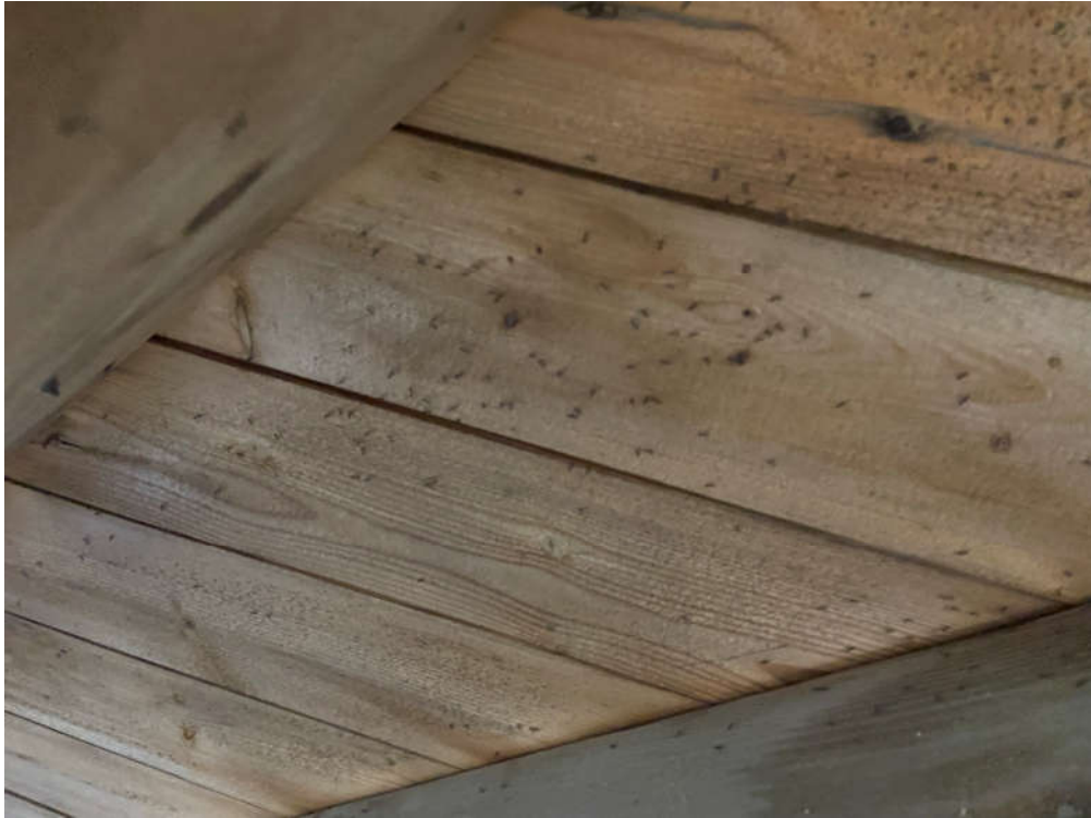
Photograph 5: Ants observed at underside of roof deck
