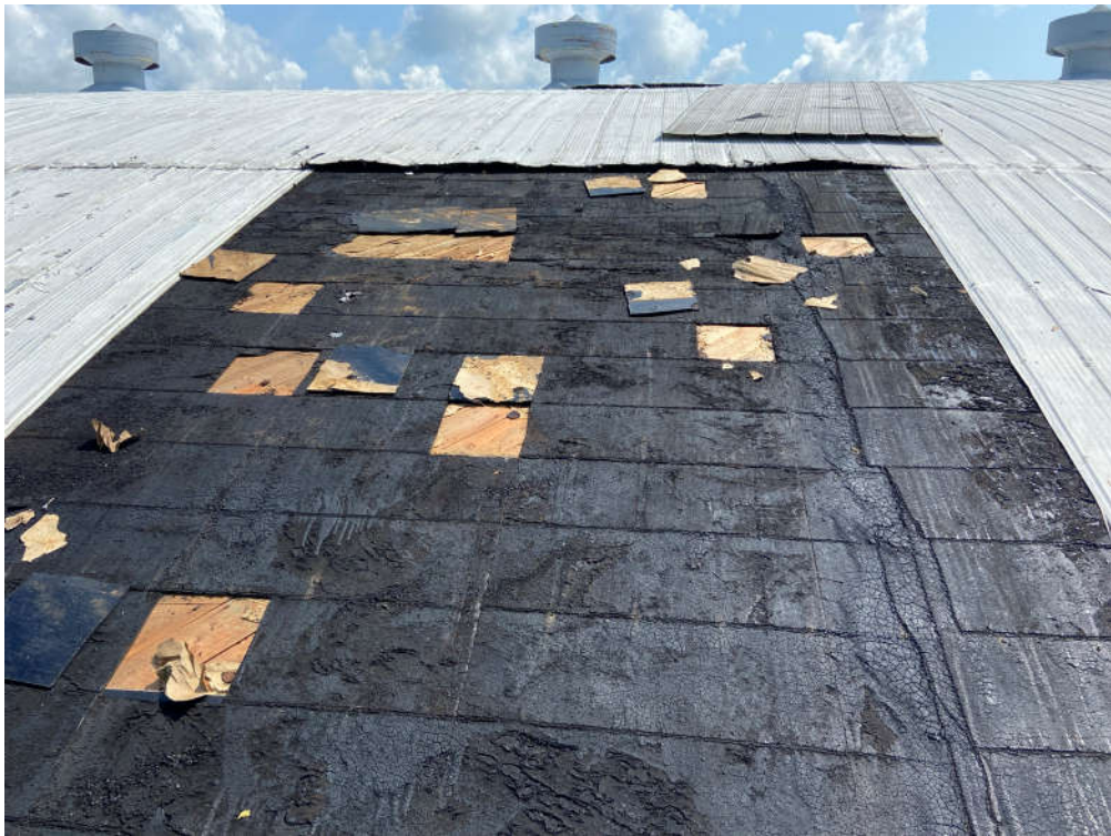
Photograph 8: Area of ant damage and deteriorated roof deck from above
