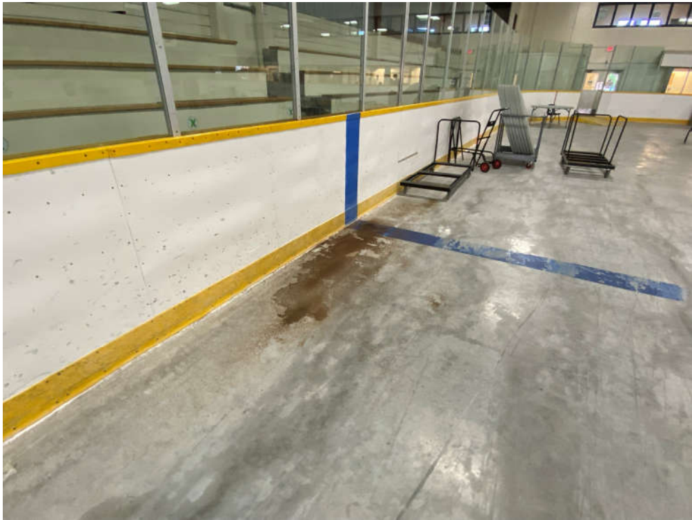
Photograph 1: Wood residue on the arena floor due to ant damage above
