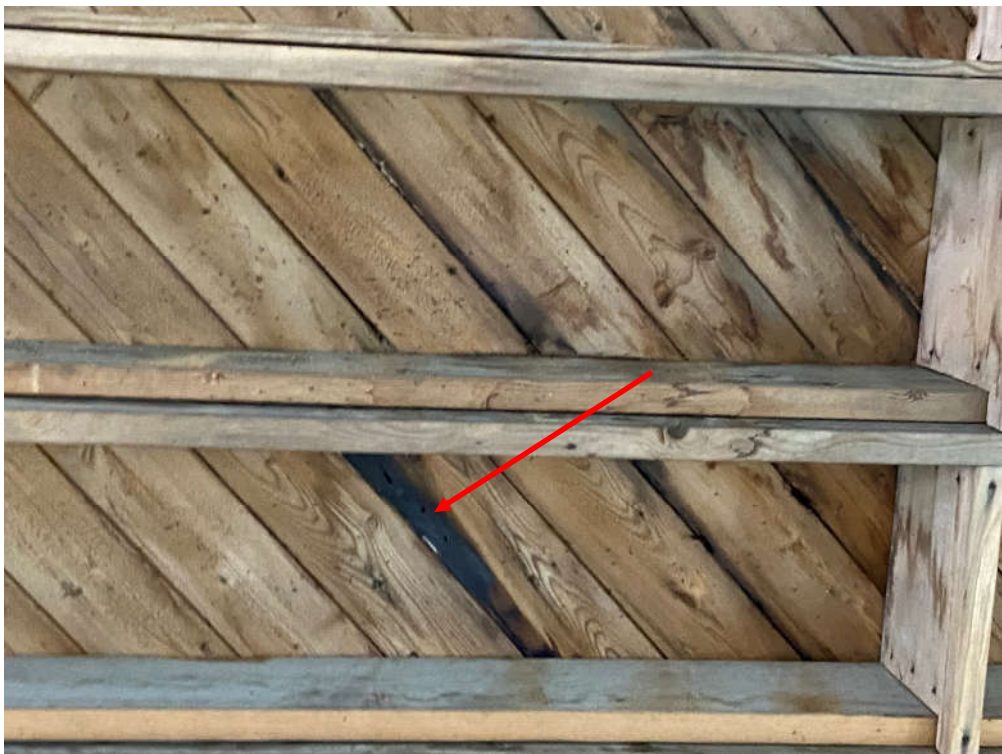
Photograph 6: Area of deck deterioration where instrument fully penetrated roof deck
