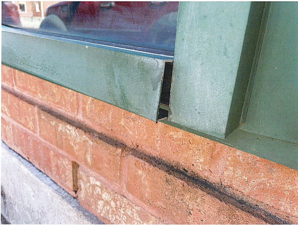
Photograph 3.1.16: Window Cap Sill Gap
