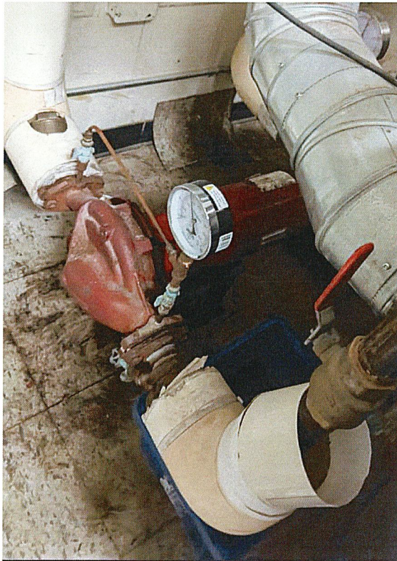
Photograph 3.2.1.4: Building Heating Loop Circulator
