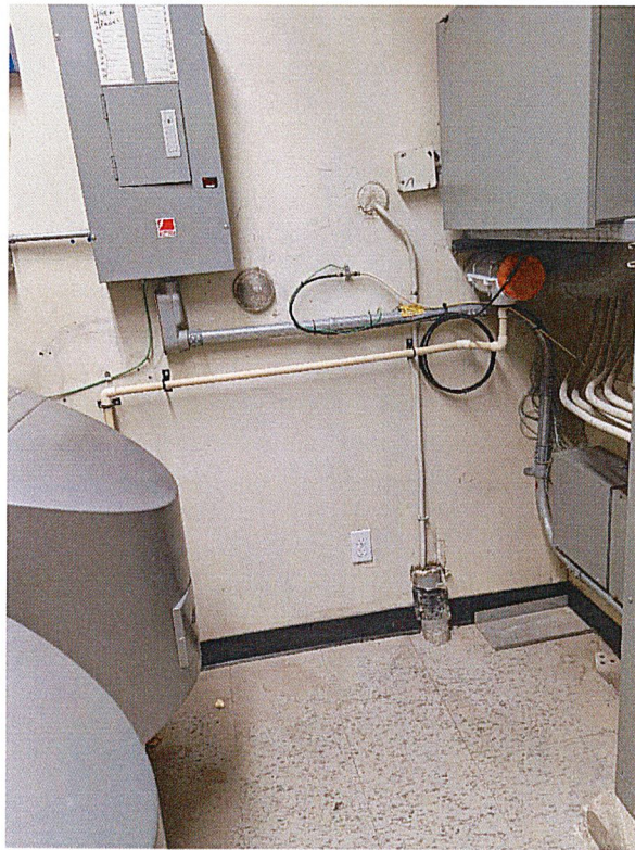
Photograph 3.3.1.3: Distribution Panel Basement
