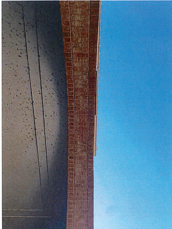
Photograph 3.1.10: Arch Deterioration - North
