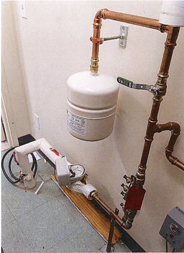
Photograph 3.2.2.2: Building Backflow Preventer
