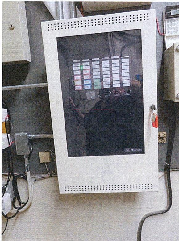
Photograph 3.3.2.2: Fire Alarm Panel
