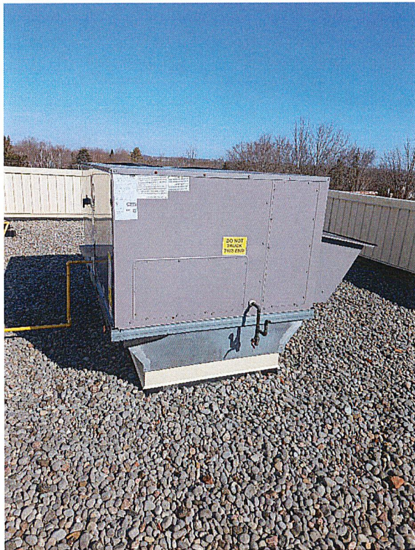
Photograph 3.2.1.7: Rooftop Unit (Typical of 4)
