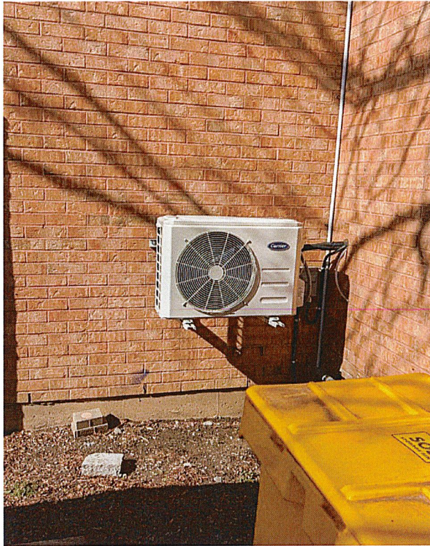
Photograph 3.2.1.6: Air Conditioner- Outdoor Unit
