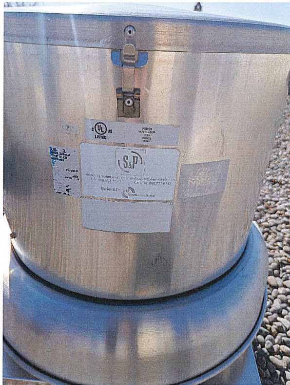
Photograph 3.2.1.8 - Washroom Exhaust Fan
