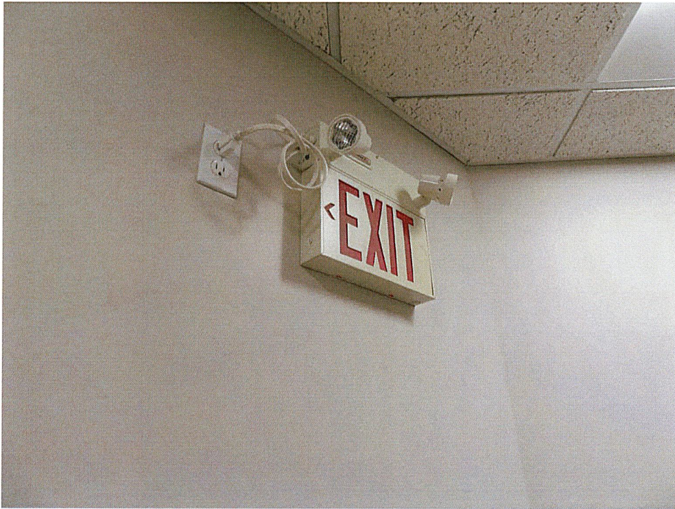
Photograph 3.3.2.1: Emergency & Exit Lighting
