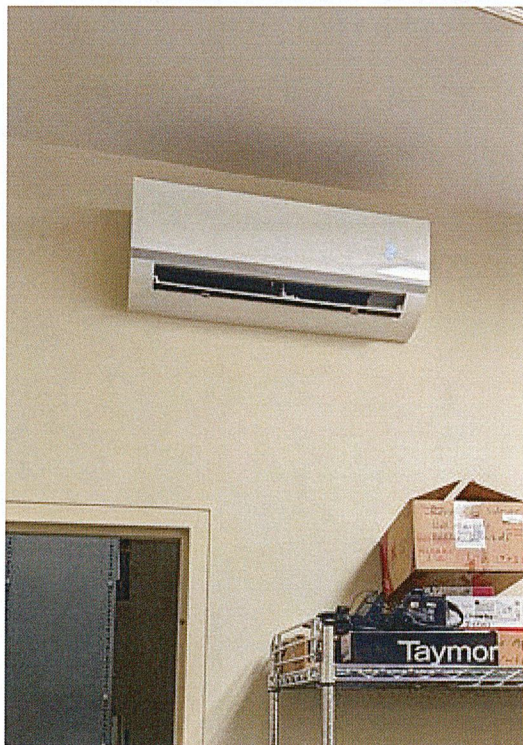
Photograph 3.2.1.5: Air Conditioner- Indoor Unit
