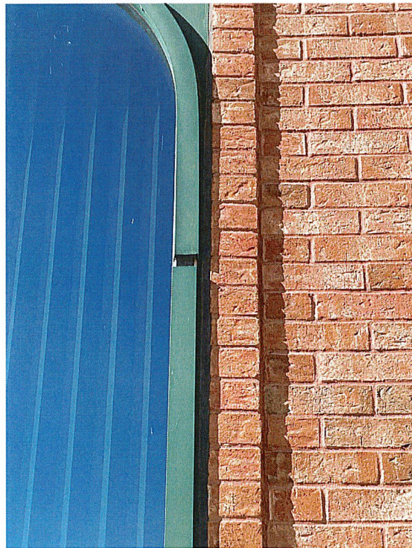
Photograph 3.1.15: Window Cap Gap
