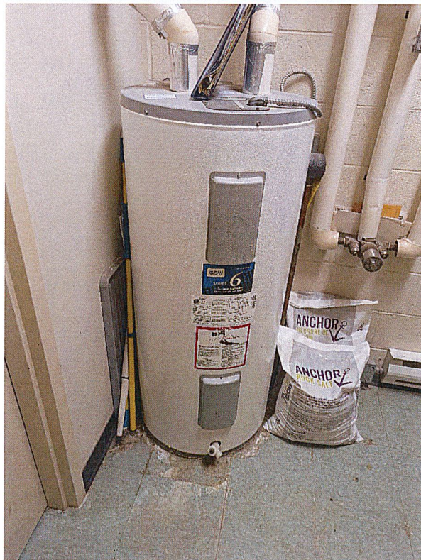
Photograph 3.2.2.1: Hot Water Tank and Mixing Valve
