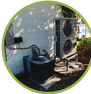
New 'Fujitsu' condenser unit installed on exterior stand
