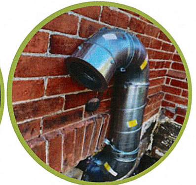
Outside air intake ductwork
