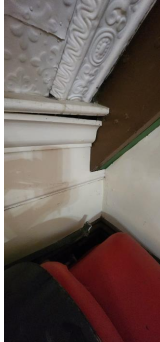
FIG. Div.9. 14 – Ceiling Crown Mold at Balcony
