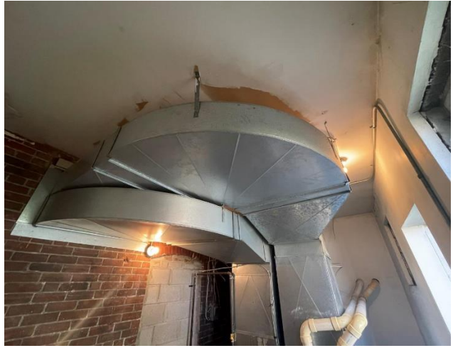
FIG. Div.15. 6 – Furnace Room 2
