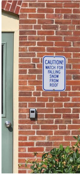
FIG. Div.2. 1- Falling Snow Warning Sign
