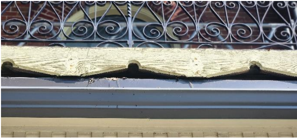
FIG. Div.6. 2 – Balcony Front Fascia
