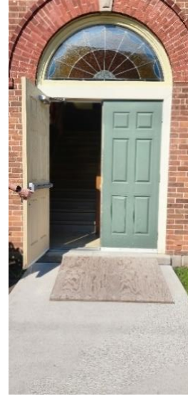
FIG. Div.8. 6 – East Exit Doors 2
