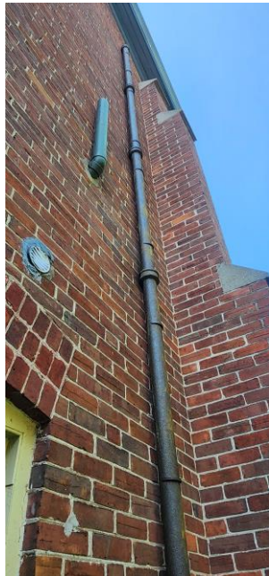
FIG. Div.15. 3 – Rear Washroom Vent Stacks and Exhaust Vent
