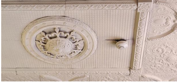
FIG. Div.9. 13 – Tin Ceiling with Detector
