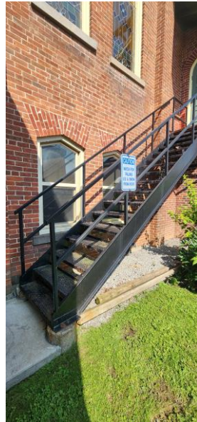
FIG. Div.5.8 - East Fire Escape 2
