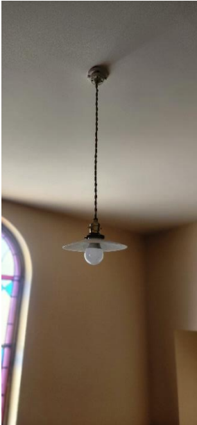
FIG. Div.16. 2 – Light Fixture Serviced by Knob and Tube Wiring
