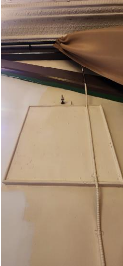
FIG. Div.5. 2 – Interior View of Anomalous Iron Through Bolt
