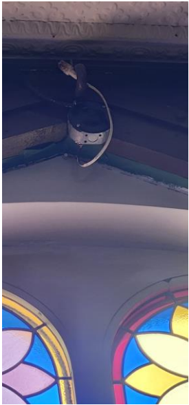
FIG. Div.16. 3 – Abandoned Fixture Outlet Box
