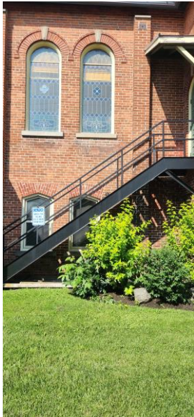
FIG. Div.5. 7 - East Fire Escape
