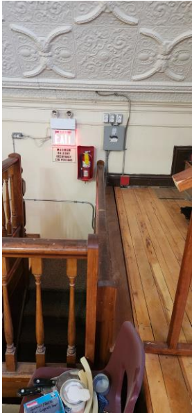
FIG. Div.16. 1 – Sub-panel at Balcony Technical Support Area
