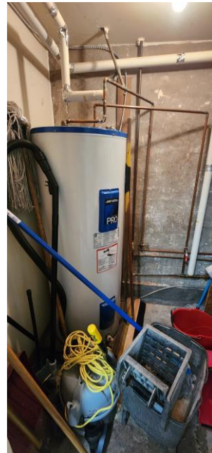
FIG. Div.15. 4 – Utility Box
