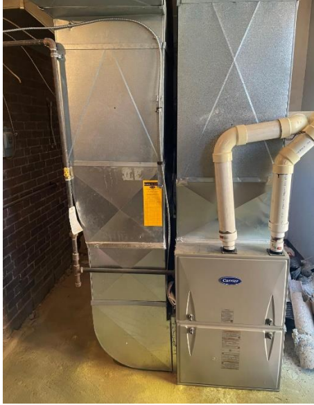
FIG. Div.15. 5 – Furnace Room 1
