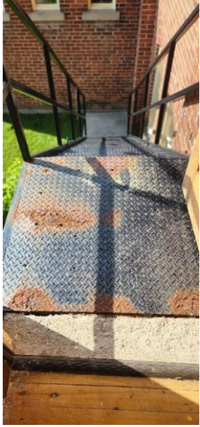
FIG. Div.5. 9- East Fire Escape Landing
