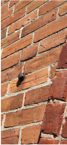
FIG. Div.5. 1 – Anomalous Iron Through Bolt at Front Wall
