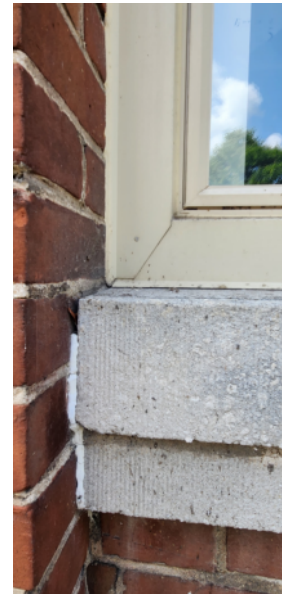
FIG. Div.3. 4 – Deteriorated Caulking Joint at Sill
