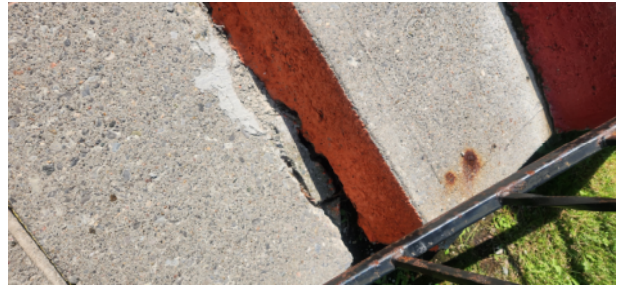
FIG. Div.2. 2 – Deterioration at Front Steps
