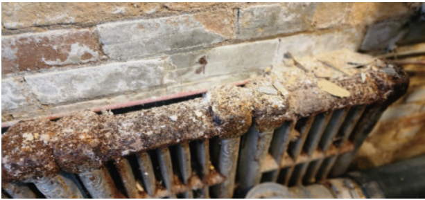
FIG. Div.4. 19 – Masonry Deterioration in Basement Due to Moisture Infiltration
