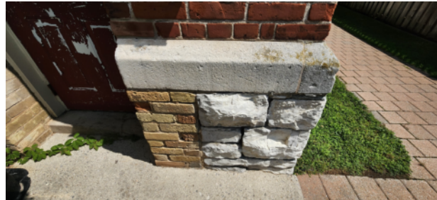
FIG. Div.4. 4 – Deteriorated Masonry Mortar Joints
