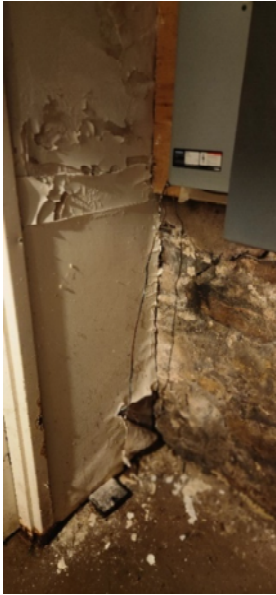
FIG. Div.9. 1 – Drywall Damage Due to Moisture Infiltration into Basement
