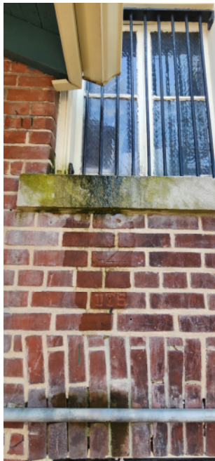
FIG. Div.4. 11 – Spill from Eave trough causing damage to masonry
