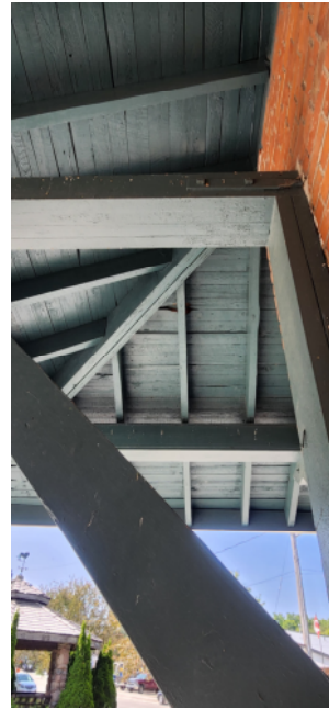
FIG. Div.6. 2 – Minor Damage to Canopy Roof Deck
