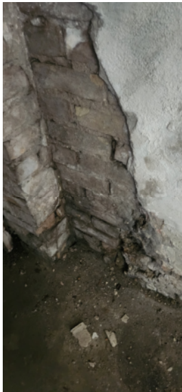
FIG. Div.9. 3 – Plaster Damage in Stair to Basement
