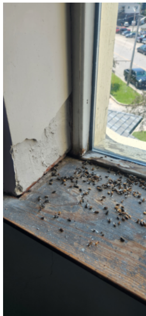
FIG. Div.9. 7 – Plaster Deterioration at Tower Stair
