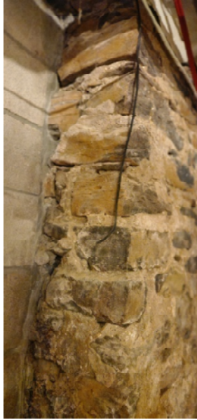
FIG. Div.4. 25 – Missing Mortar in Original Rubble Stone Foundation
