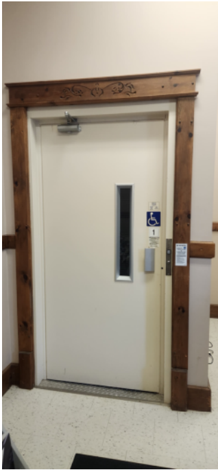
FIG. Div.14. 1 – Personal Accessible Lift (PAL) Connecting Main Floor to Auditorium Above
