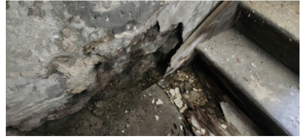
FIG. Div.4. 28 – Damage to basement foundation and stair due to moisture infiltration
