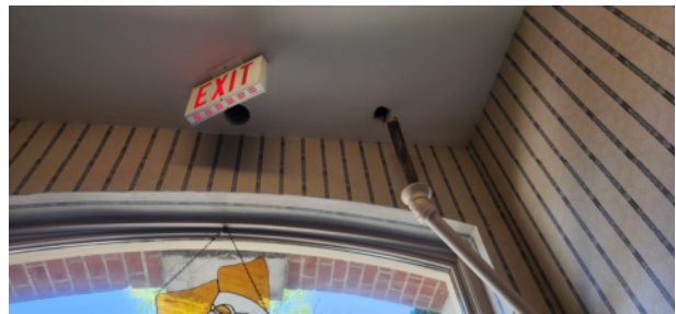
FIG. Div.15. 8 – Disconnected Vent Pipe
