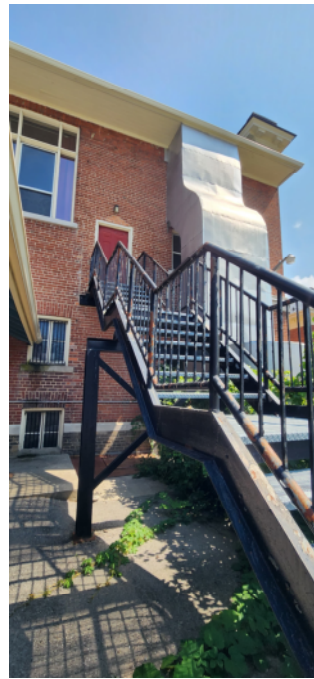
FIG. Div.5. 2 – Corrosion of Metal Fire Escape
