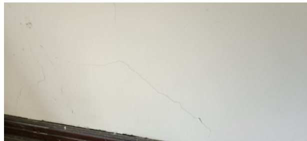
FIG. Div.9. 8 – Plaster Delamination at Tower Stair
