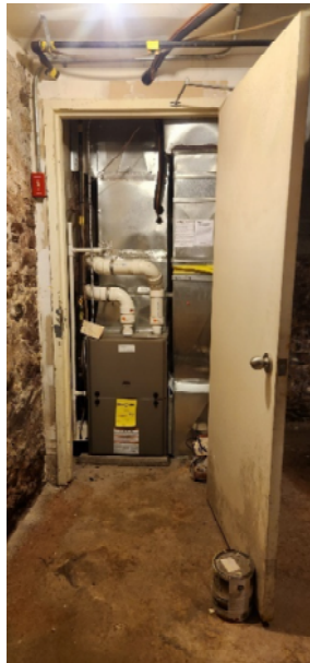
FIG. Div.15. 3 – Second of Two Furnace Rooms
