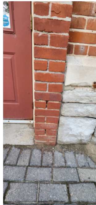
FIG. Div.4. 8 – Deteriorated Mortar Joints
