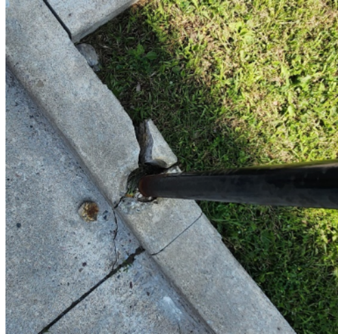
FIG. Div.2. 6 – Rusting Handrail Post Spalling Concrete Curb
