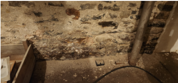
FIG. Div.4. 27 – Deteriorating Masonry Joints
