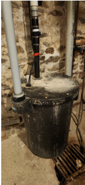
FIG. Div.15. 7 – Existing Sewage Sump Pump
