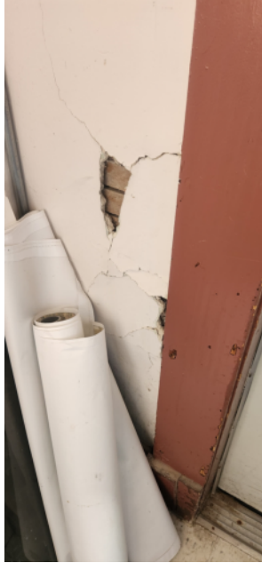
FIG. Div.9. 5 – Plaster Damage in Auditorium Exit Stair
