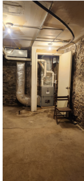
FIG. Div.15. 2 – Furnace Room
