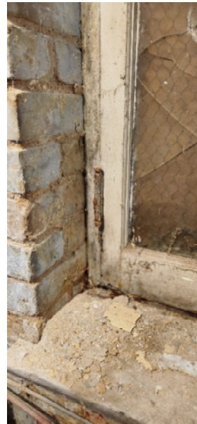
FIG. Div.4. 20 – Masonry Deterioration in Basement Due to Moisture Infiltration 3 @ Window Well
