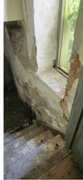
FIG. Div.4. 26 – Evidence of Moisture Infiltration at Stair to Basement
