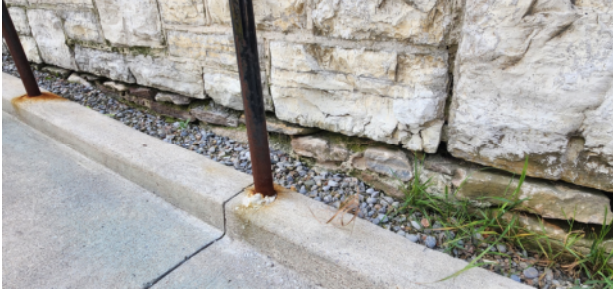
FIG. Div.4. 1 – Loss of Mortar Adjacent to Ramp
