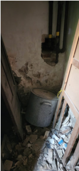
FIG. Div.9. 4 – Damage and Debris in Stair to Basement
