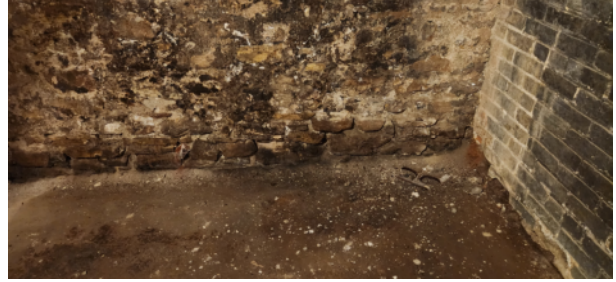
FIG. Div.4. 22 – Deteriorating Mortar in Rubble Foundation Wall
