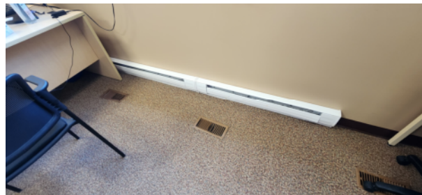
FIG. Div.15. 4 – Two Separate Heating Systems in Ontario Works Office
