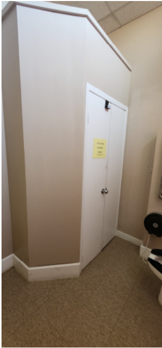
FIG. Div.14. 2 – Elevator Machine Room
