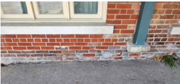
FIG. Div.4. 3 – New Precast Concrete Window Sill and Deteriorated Masonry Below
