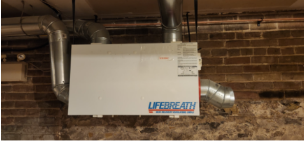
FIG. Div.15. 5 – Energy Recovery Ventilator
