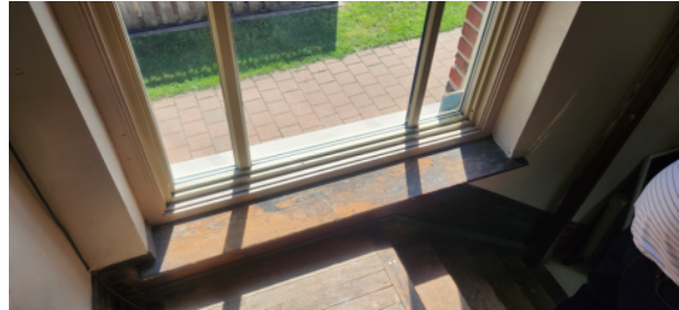
FIG. Div.9. 6 – Some Deteriorated Plaster at Window Surround in Auditorium Stair
