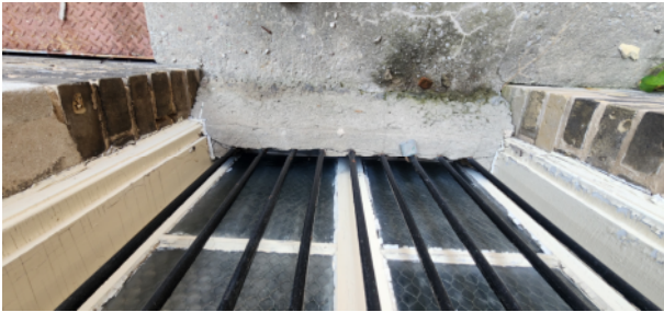
FIG. Div.3. 1 – Concrete Patching at Window Well
