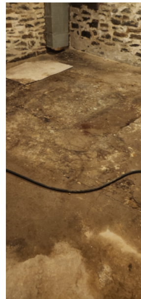
FIG. Div.4. 24 – Evidence of Moisture Infiltration at Basement Floor
