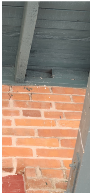
FIG. Div.6. 3 – Minor Damage at Canopy Roof Deck Crown Mold
