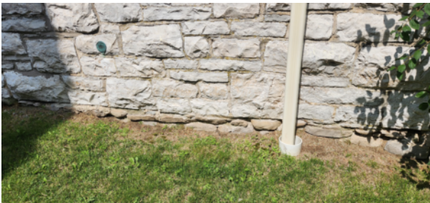
FIG. Div.4. 7 – Deteriorated Mortar Joints at Grade
