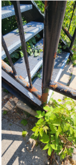
FIG. Div.5. 1 – Detail of Metal Corrosion on Fire Escape
