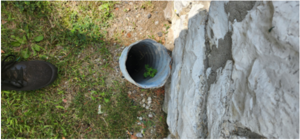
FIG. Div.2. 1 – Abandoned Downspout Drain
