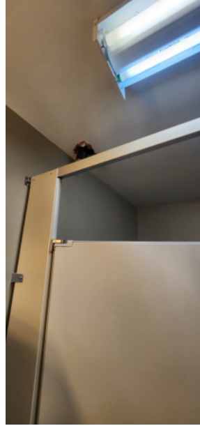
FIG. Div.9. 14 – Drywall Ceiling Damage in Washroom
