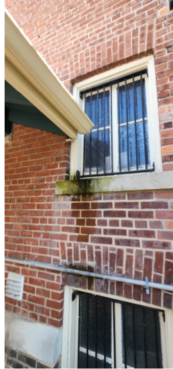
FIG. Div.4. 10 – Water Damage at Eave trough Overflow
