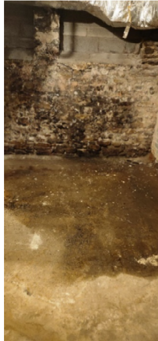
FIG. Div.4. 30 – Evidence of Water Infiltration on Floor Slab
