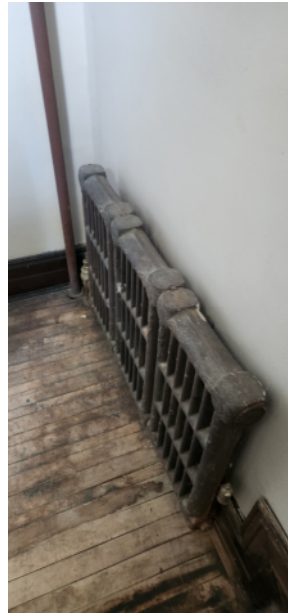
FIG. Div.15. 6 – Obsolete Radiator at Stair to Basement
