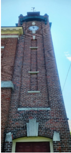
FIG. Div.4. 17 – Beaverton Hall Tower Indicating Different Coloured Bricks
