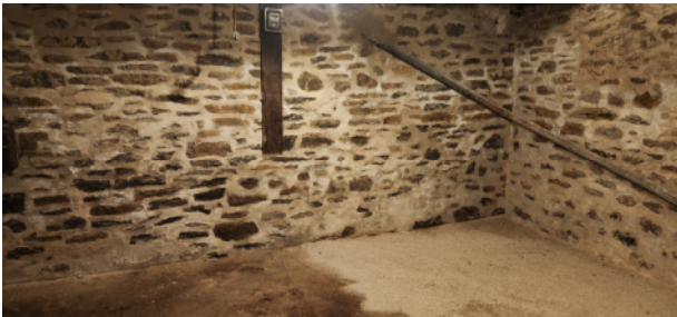
FIG. Div.4. 23 – Restored Masonry Joints in Area that Still Exhibits Moisture Infiltration
