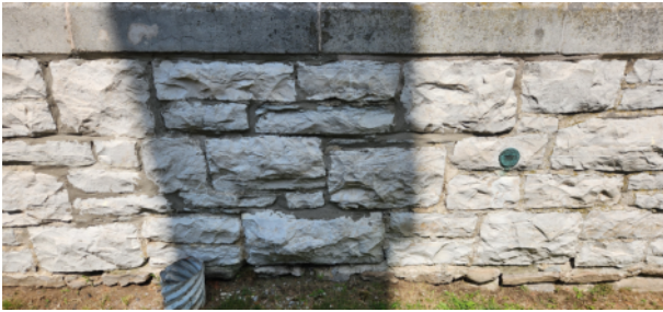
FIG. Div.4. 9 – Non-compatible Mortar Repairs
