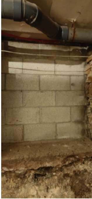
FIG. Div.4. 29 – Evidence of Moisture Infiltration at Basement
