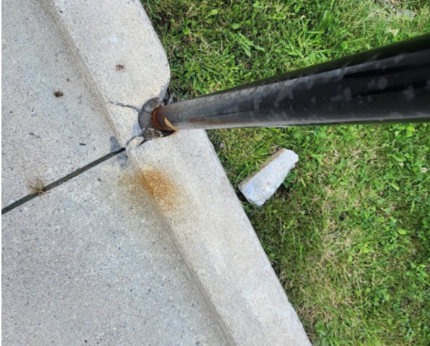
FIG. Div.2. 5 – Rusting Handrail Post Spalling Concrete Curb
