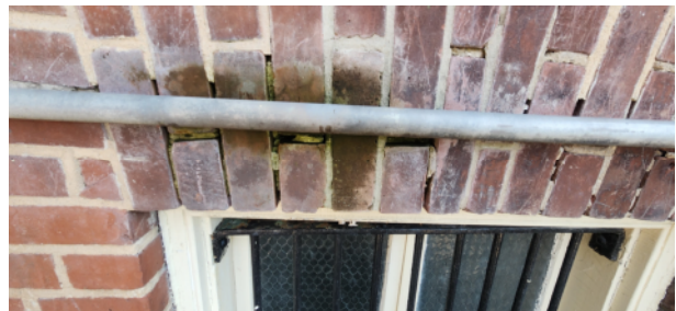
FIG. Div.4. 12 – Deteriorating Mortar Joints at Window Arch
