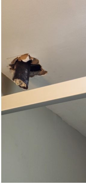
FIG. Div.9. 13 – Projecting Pipe at Washroom Ceiling
