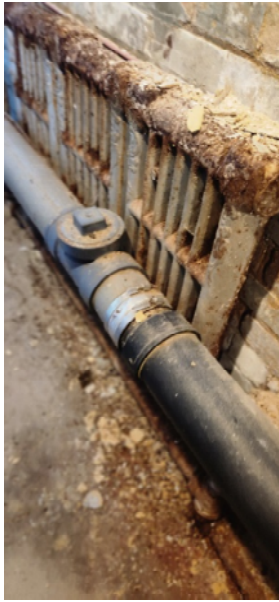
FIG. Div.4. 21 – Masonry Deterioration in Basement Due to Moisture Infiltration 2
