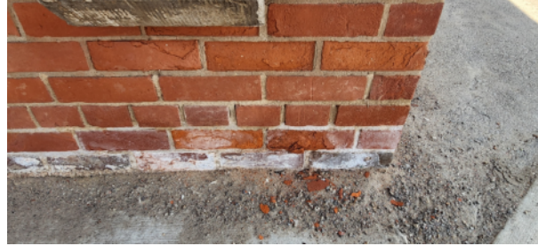
FIG. Div.4. 2 – Masonry Deterioration due to De-icing Salts
