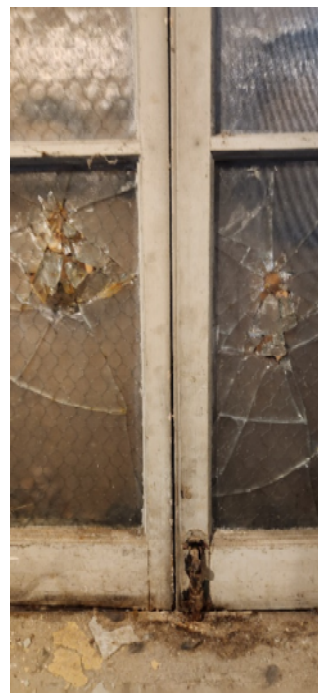
FIG. Div.8. 4 – Basement Window Damage
