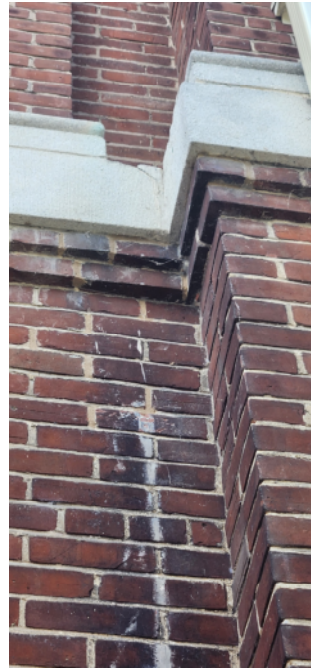
FIG. Div.3. 6 – Crack in Roman Stone Banding
