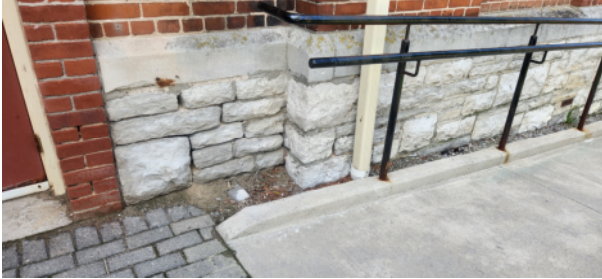
FIG. Div.4. 5 – Loss of Mortar at Front Entrance
