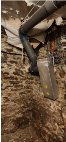
FIG. Div.9. 2 – Deteriorated Fire Separation at Ceiling in Basement
