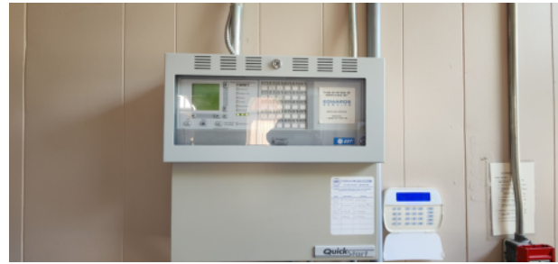
FIG. Div.16. 2 – Fire Alarm and Security Alarm Panels
