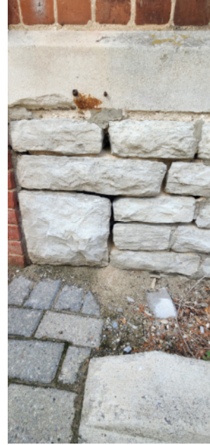
FIG. Div.4. 6 – Deteriorated Mortar Joints
