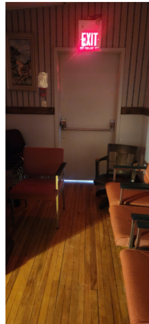
FIG. Div.8. 8 – Auditorium Balcony Access to Exit Blocked by Furniture
