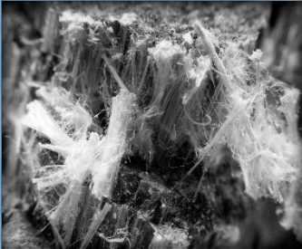
Asbestos in Buildings
