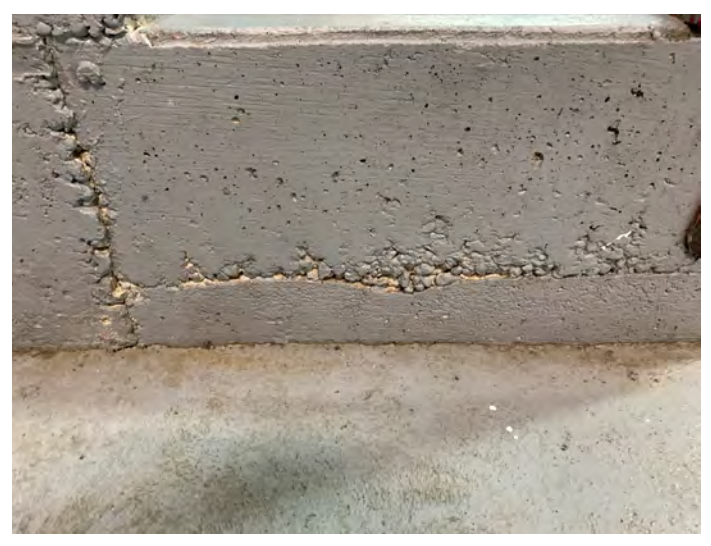
Photo 16 - Bleacher Seating Honeycombing
