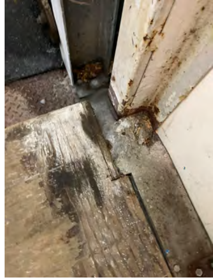
Photo 30 - Concrete Apron Slab Efflorescence
