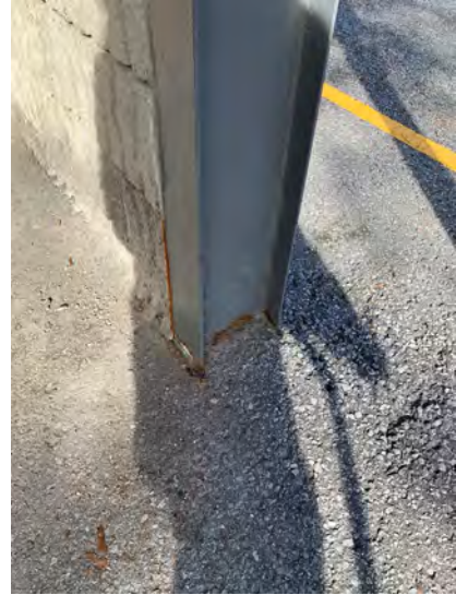
Photo 54 - West Elevation Exterior Column Base Corrosion
