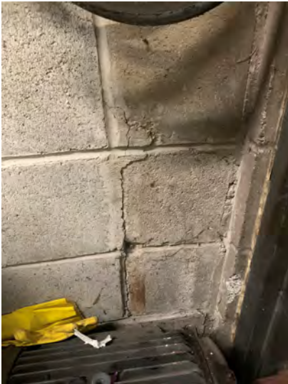
Photo 27 - Masonry Block Wall Cracking
