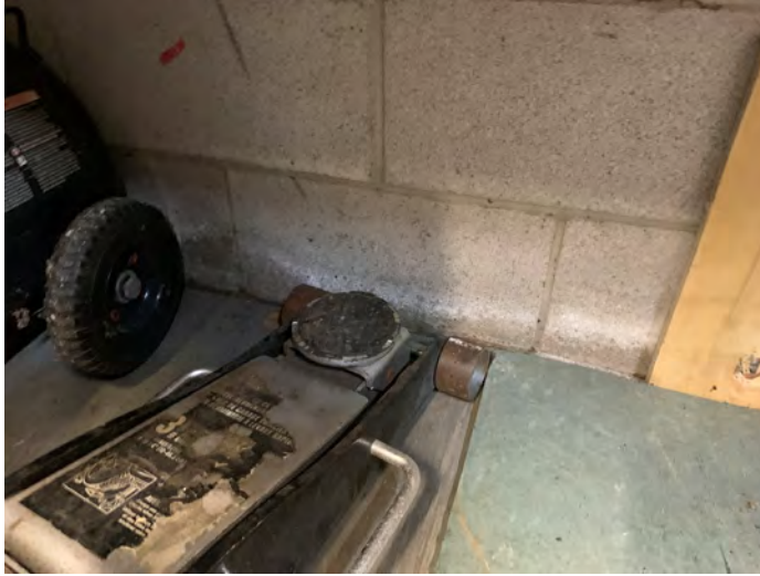
Photo 21 - Masonry Block Wall Efflorescence
