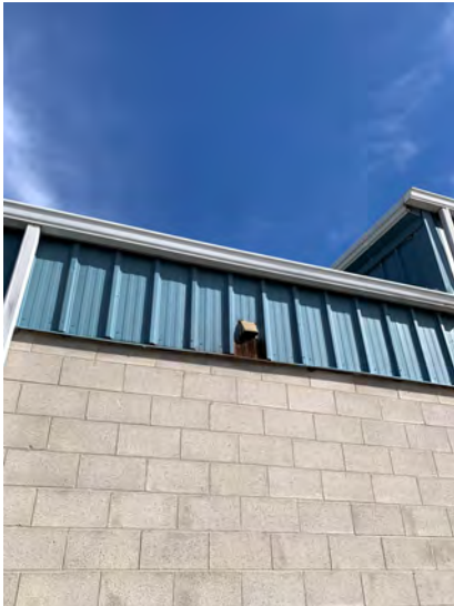
Photo 47 - North Elevation Corroded Cladding
