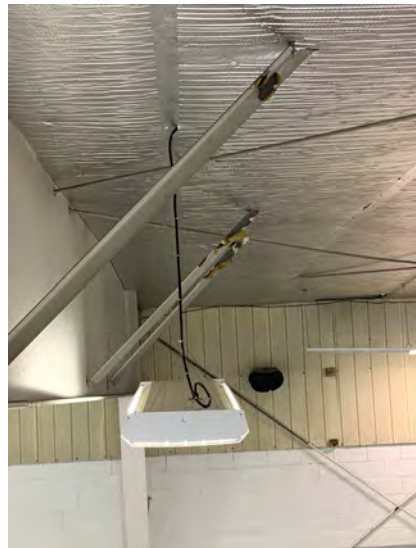
Photo 12 - Pre Engineered Frame Bridging Peeling
