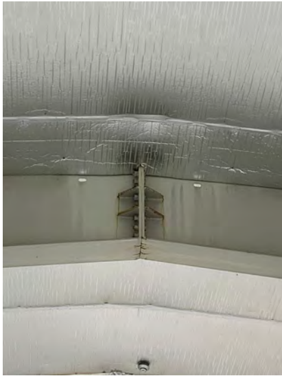
Photo 09 - Pre Engineered Frame Moisture Staining
