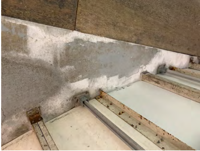
Photo 29 - Concrete Apron Slab Efflorescence
