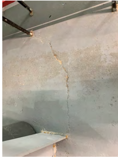
Photo 18 - Bleacher Seating Cracking
