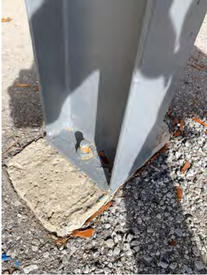
Photo 53 - West Elevation Exterior Column Bolted Connection Corrosion
