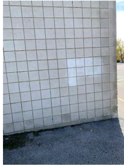
Photo 44 - East Elevation Block Wall Efflorescence
