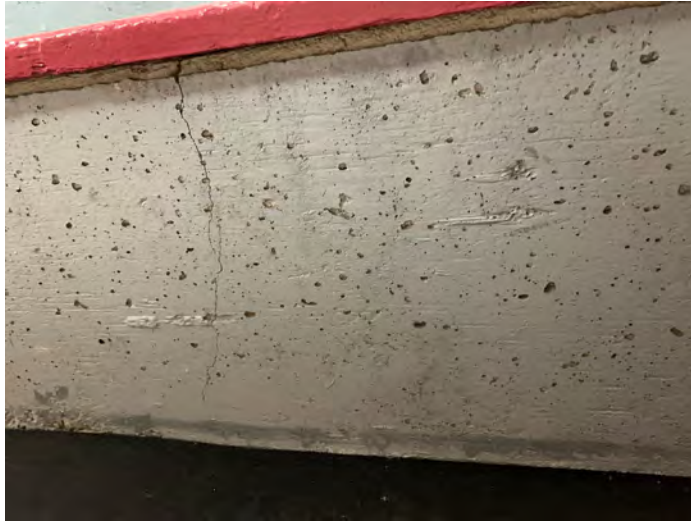
Photo 17 - Bleacher Seating Minor Cracking
