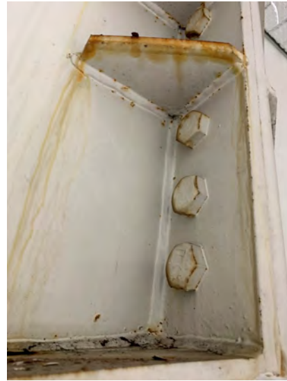
Photo 06 - Pre Engineered Frame Bolted Connection Corrosion
