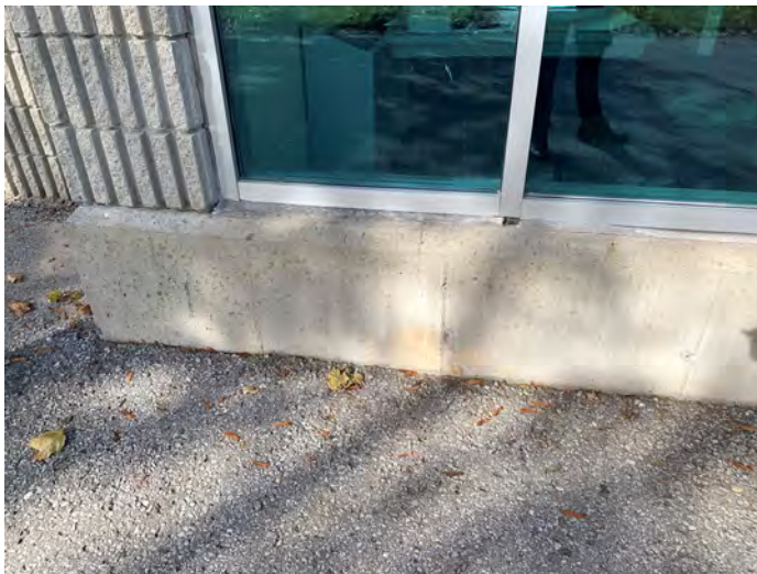
Photo 55 - West Elevation Foundation Wall Vegetation and Efflorescence
