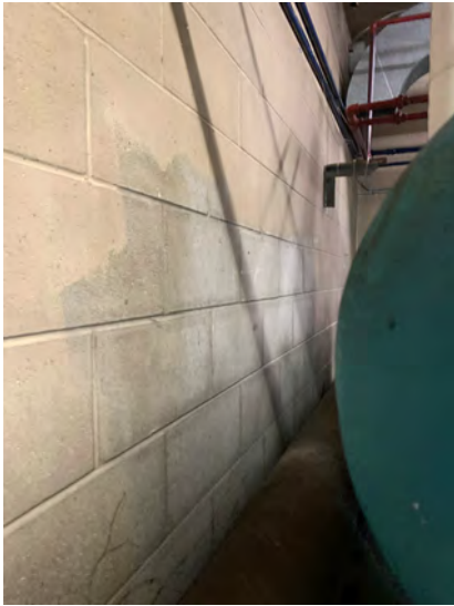
Photo 25 - Masonry Block Wall Deterioration
