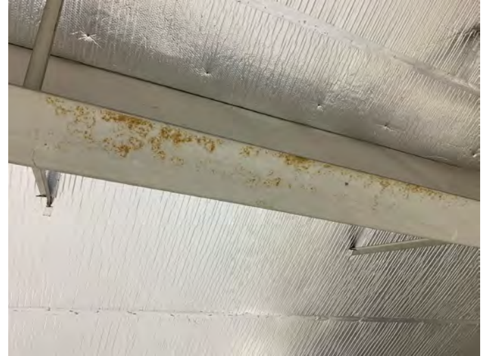
Photo 02 - Pre Engineered Frame Bottom Flange Corrosion
