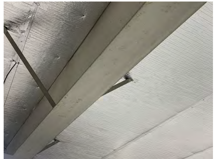
Photo 04 - Pre Engineered Frame Bottom Flange Corrosion
