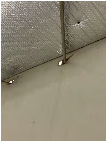
Photo 15 - Pre Engineered Frame Bracing Corrosion
