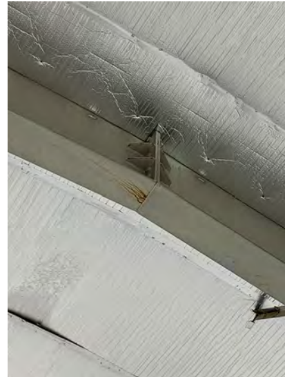
Photo 08 - Pre Engineered Frame Moisture Staining
