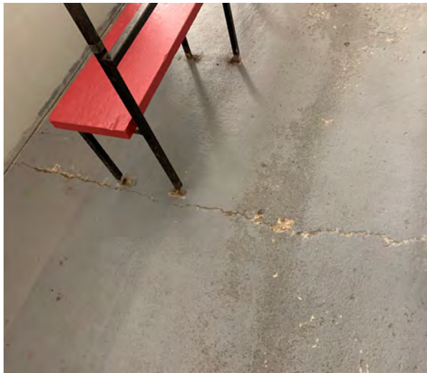
Photo 19 - Bleacher Seating Cracking
