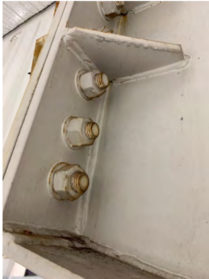
Photo 07 - Pre Engineered Frame Bolted Connection Corrosion
