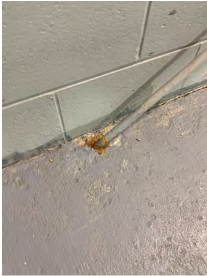
Photo 13 - Pre Engineered Frame Bracing Corrosion
