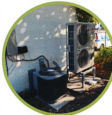
New 'Fujitsu' condenser unit installed on exterior stand
