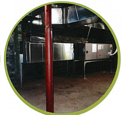
Associated indoor heat pump unit mounted on interior stand
