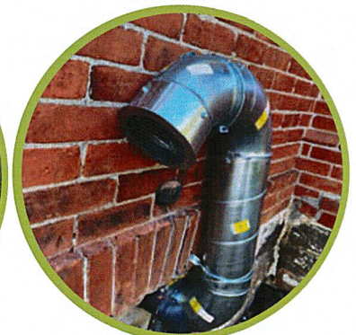
Outside air intake ductwork
